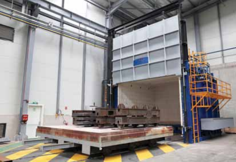
New Heat Treatment Furnace
